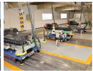
MX-30 EV battery charging stations
