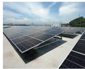
Hiroshima Plant's rooftop solar panels
